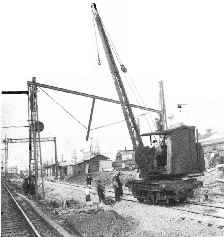
Special Works gang erects overhead structures on the new track between Burnley and Richmond.
