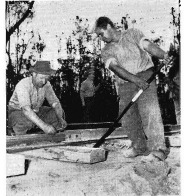
(From left) L. H. Platelayer F. S. Roczynski and P. Chila are preparing to cut in the last rail on a deviation.
