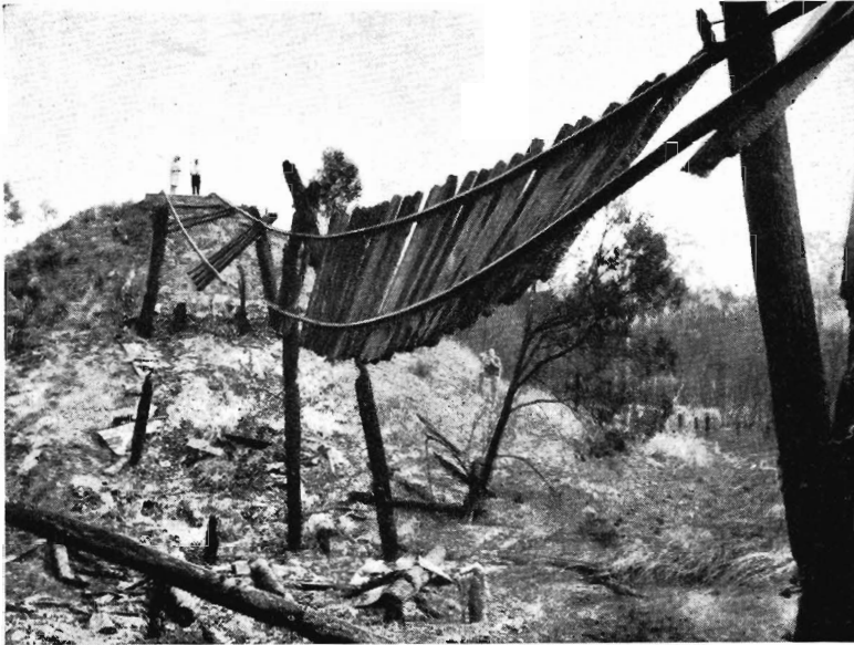
Fire twisted remains of bridge over Dirty Hollow Creek ("The Age" photograph)
