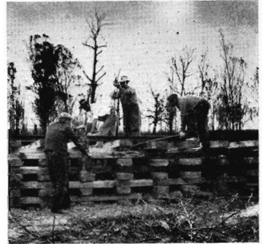
(Left to right) J. Butaskas, M. Jojic (Ganger), L. Skeen, and W. Rudewicz build a "pig sty"—a temporary support for the track to replace a burnt bridge.
