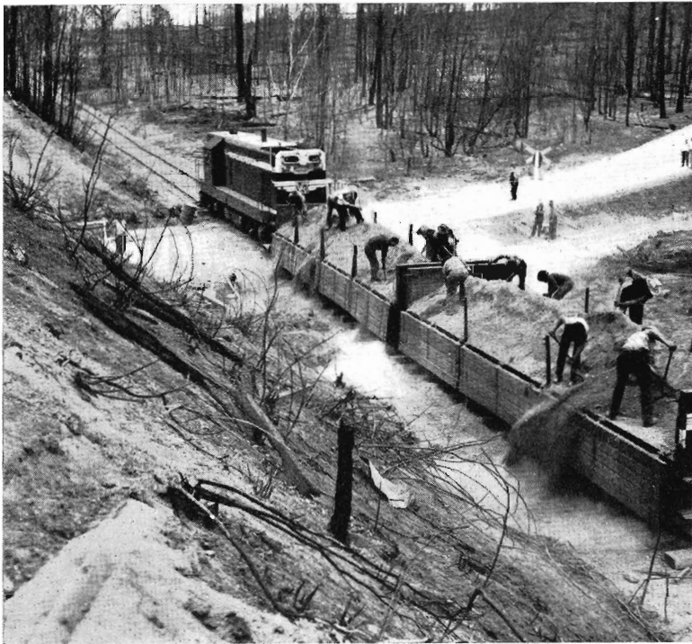
A ballast train is being unloaded at the deviation that temporarily replaced the rail bridge over the Swan Reach-Mossiface Road.
