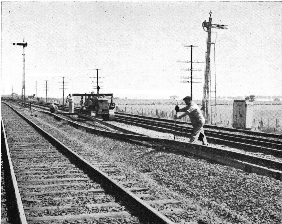
A platelayer bars out the old rail over the new rail. Behind him, a crawler tractor with suspended rail threader is slewing the new rail into position. The 225 ft. rails have been joined with fishplates into lengths of up to half a mile. The threader lays them at the rate of about one chain a minute.
