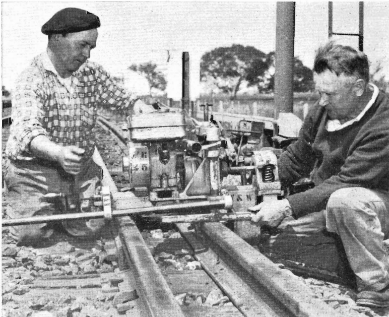
Rail boring machine is drilling holes for fishbolts in new rail of special length.
