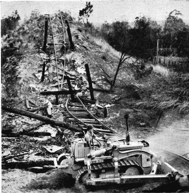
Bulldozer Operator R. Hobson clears away debris of burnt bridge over Dirty Hollow Creek.
